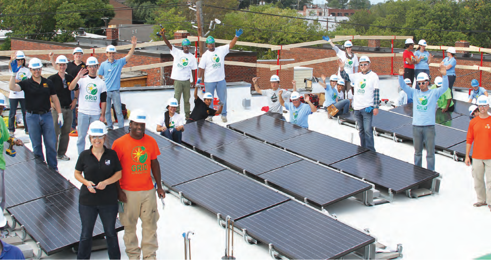
An aggressive commitment to rooftop solar installations in Los Angeles will expand the local economy, accelerate the transition to clean energy, and lead to dynamic job growth.
